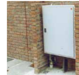
Six meter cabinet
