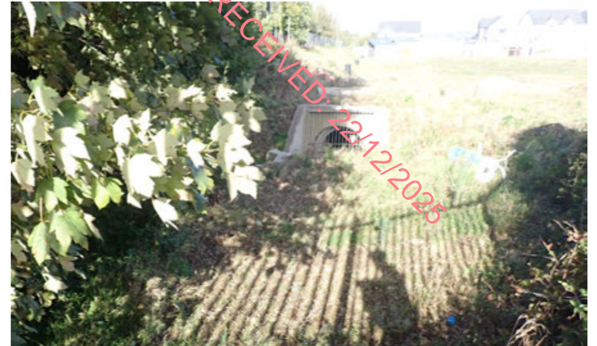
Photo 9.3.27 – View of surface water storm drain system that connects to the Ballyowen Stream. This is located in the west end of the field on the south side of the school. It is proposed that the sites stormwater discharge would connect to this system.
