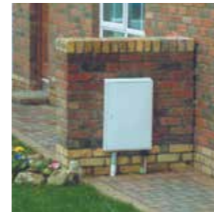
Domestic meter box
