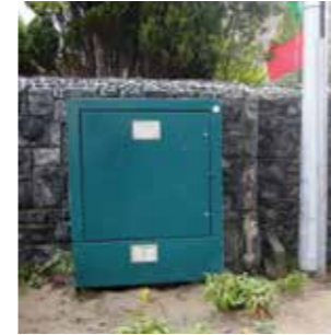
District Regulating Installation (DRI)
